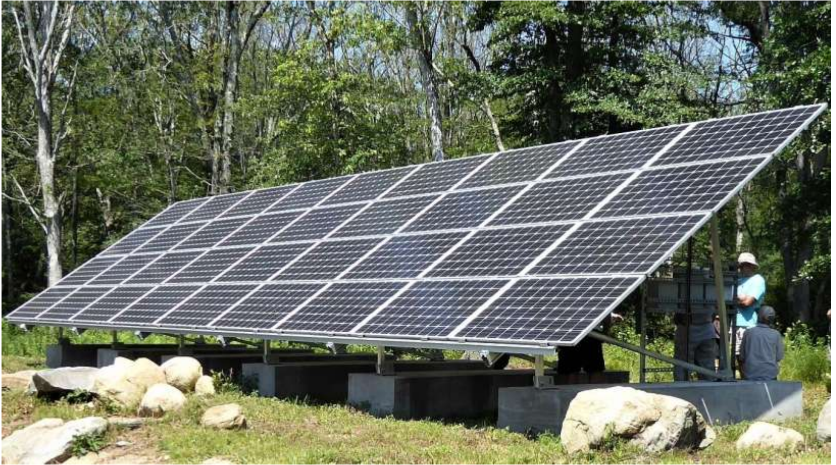
Photovoltaic panel system for a high hoop farm in North Kingstown RI
